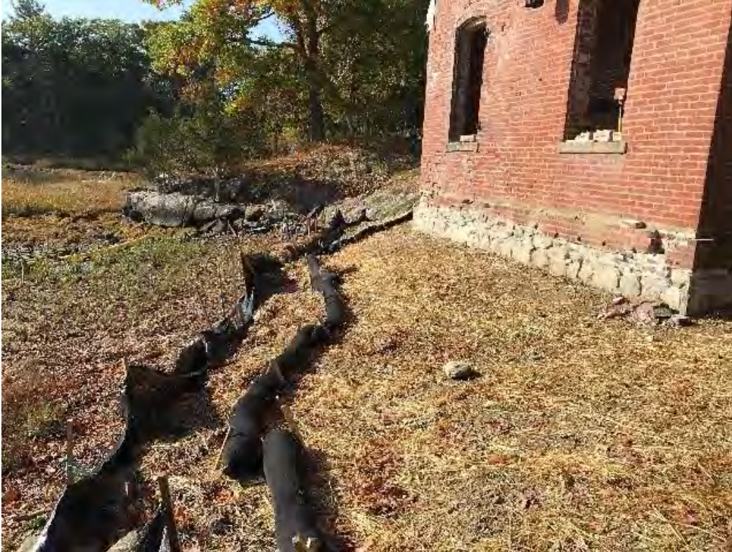
Fig 7: Toe of the slope below the cable house at Eversource property/west side of the bay. Viewing south. (10-07-20)
