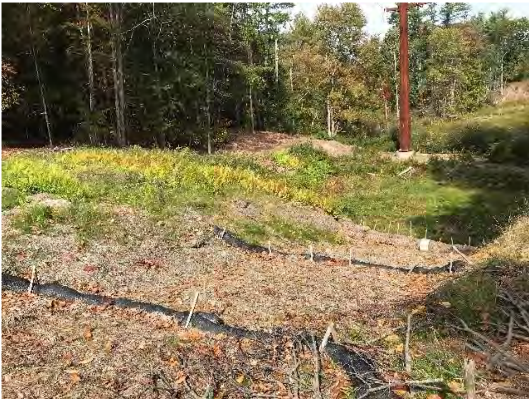
Fig 10: The slope between Strs. 28 and 29. Viewing northwest. (10-07-20)
