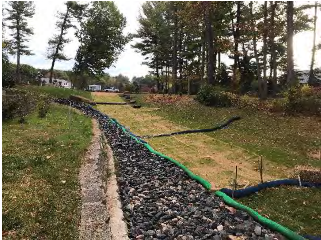
Fig 2: The slope above the manhole at Gundalow Landing/east side of the bay. Viewing east. (10-07-20)
