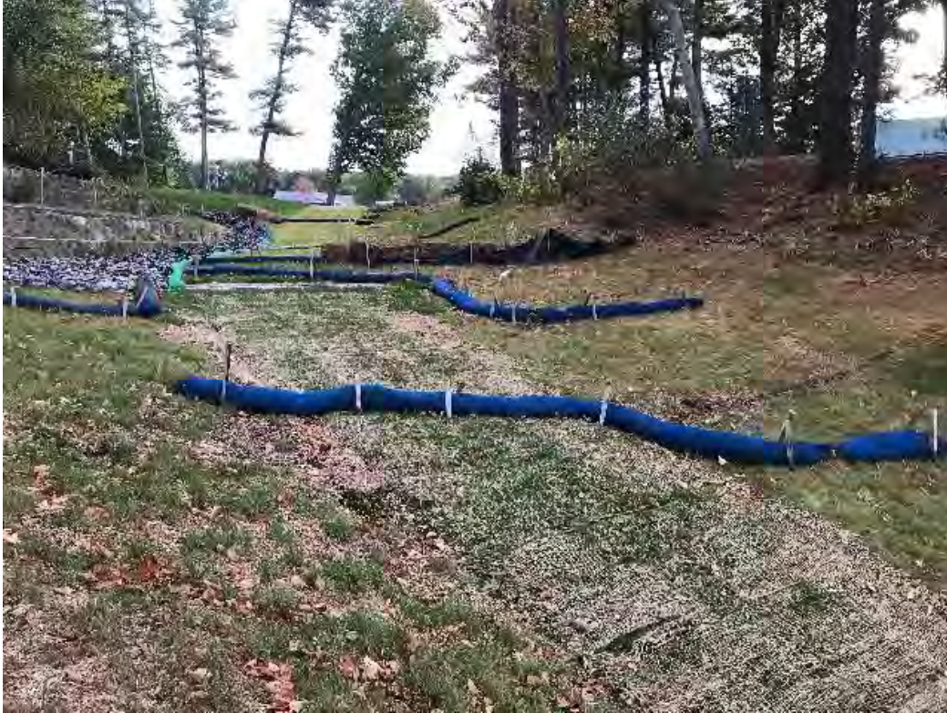
Fig 3: Slope below the manhole at Gundalow Landing/east side of the bay. Viewing east. (10-07-20)
